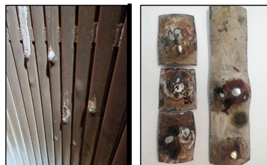
Fig. 6. “Caustic corrosion” of water heating pipes and samples of defective pipes
